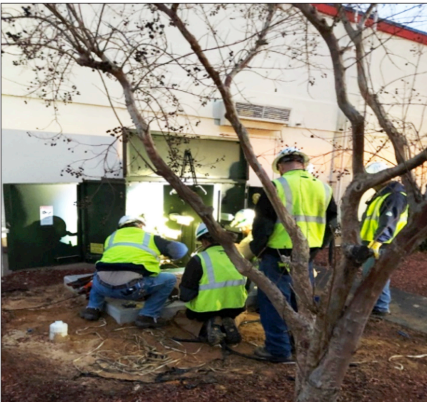
FIGURE 1: Sandhills linemen installing the three-phase GER into an existing 150 kVA padmount transformer at Fort Bragg
