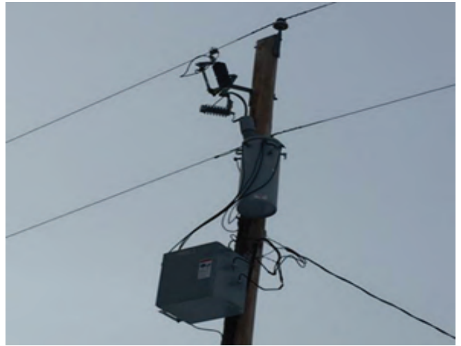
Grid Energy Router installed next to the distribution transformer.
