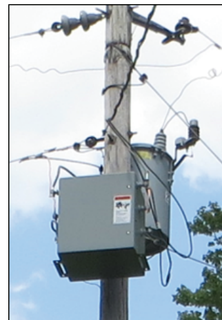
GridBridge GER installed to maintain customer voltage quality during peak demand reduction events.
