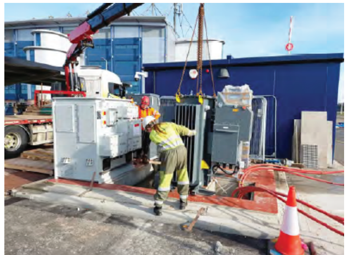
In late October, Scottish Power Energy Networks (SPEN) completed the installation of their LV Engine at Falkirk Soccer Stadium in Scotland, incorporating the Unified Power Flow Controller (UPFC) developed by ERMCO-GridBridge. The selection of GridBridge, ERMCO’s Research and Development Center in Raleigh, North Carolina, to lead SPEN’s LV Engine Program occurred in 2019. Following this, in November 2023, SP Energy Networks, a partner of GridBridge, and their Future Networks team garnered multiple accolades at the Institution of Engineering and Technology (IET) International Excellence and Innovation Awards. Notably, the LV Engine secured a gold medal in the Power and Energy category.
